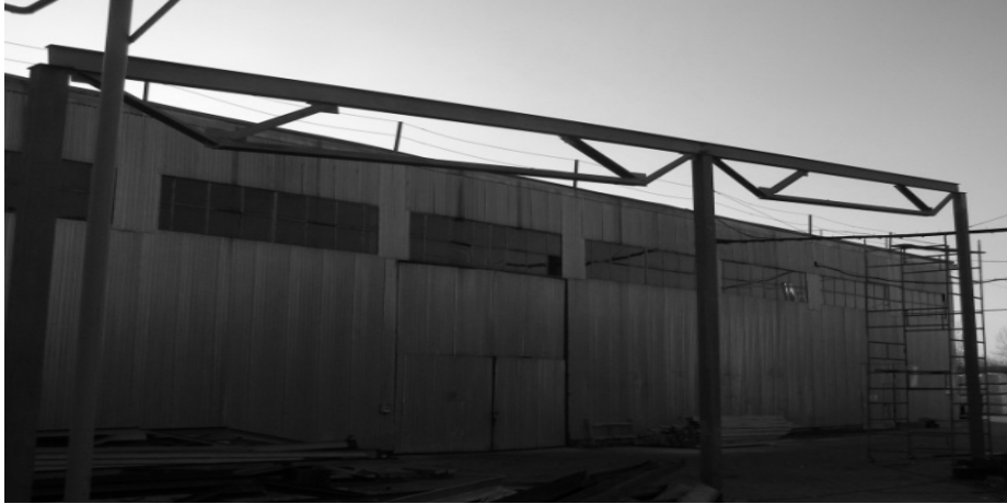
Fig. 5. Little Farm overlapping element combined with adjustment effort L = 12 m. Plant "Carpathian Ceramics" c. Kalush, Ivano-Frankivsk oblast., 2011
