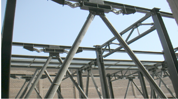
Fig. 8. Steel structure of industrial facility with V-shaped friction dampers
